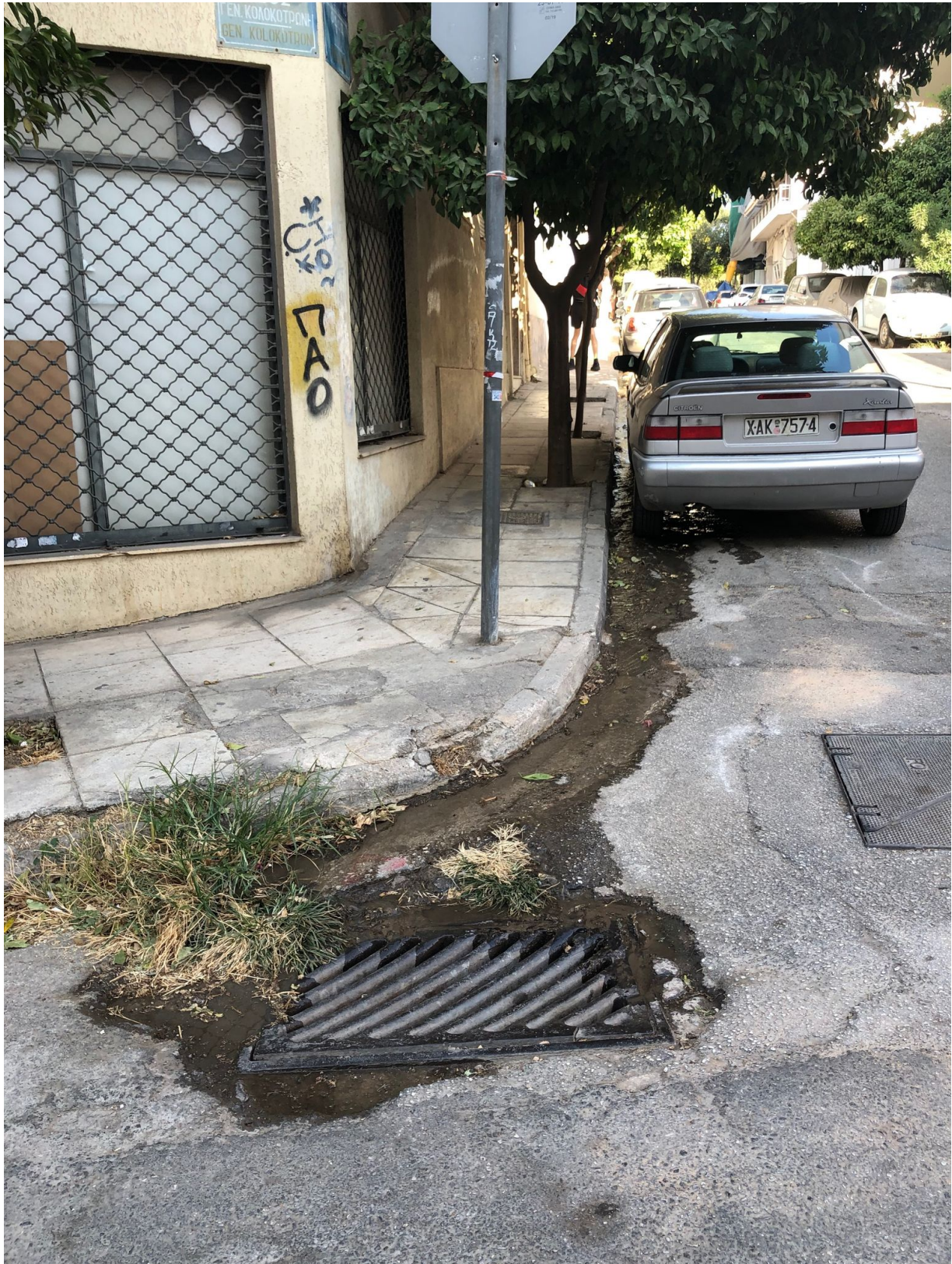
Condensed water running down the street from the air conditioning or something another? Authors' archive.
